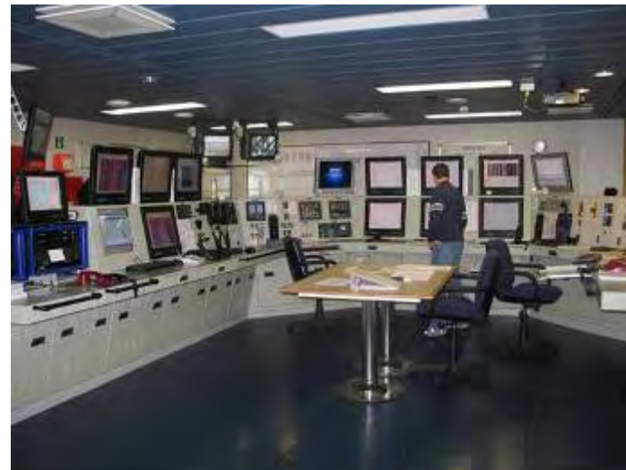
Central Control Room
